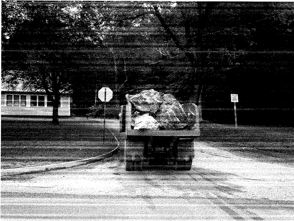
September 5, 2011: FWW rock truck hauling ledge stone to large river bank erosion
