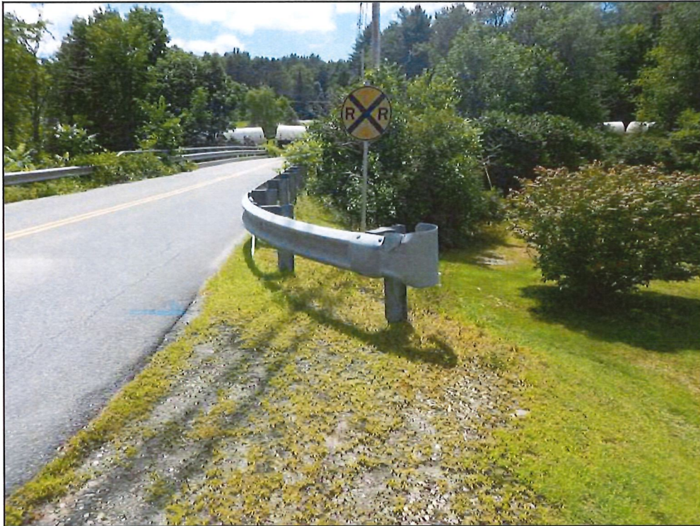
Photo 8. Photo shows the road fill and sloping ground on the northwest quadrant of the bridge over the Williams River. A train traversing the Rutland and Burlington Railroad is visible in the background. View is to the southwest.
