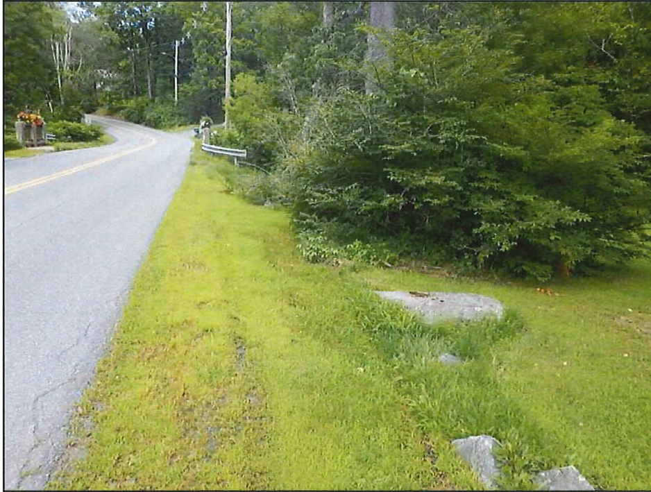
Photo 3. Photo shows the drainage ditch and fill on the east side of Church Street directly south of the Lovers Lane bridge. The bridge railings are visible on the left. The upward slope of Church Street is visible in the background. View is to the north.
