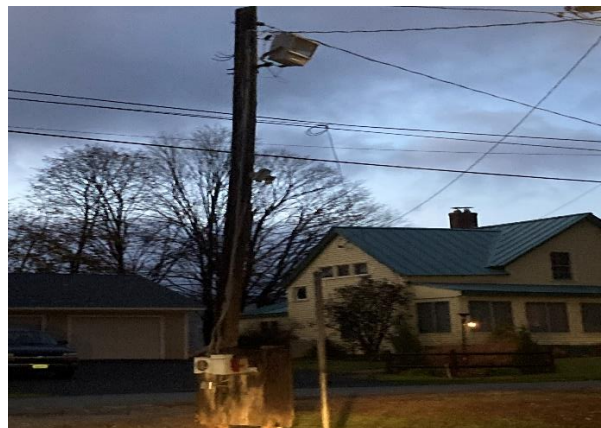
Abandoned light pole and electric meter
