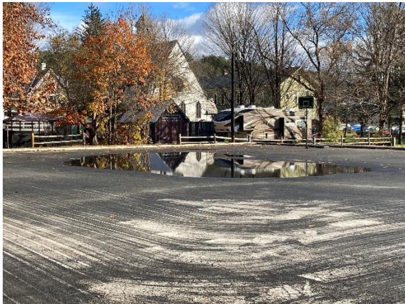
Ice rink surface that doesn't drain storm water
